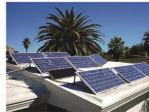
Solar PV System
